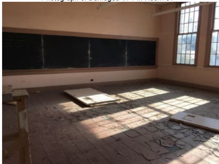
Photograph of Damaged VFT in Room 31
